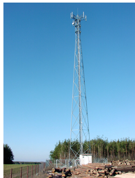
Figure 1: GSM broadcasting station – real photo
