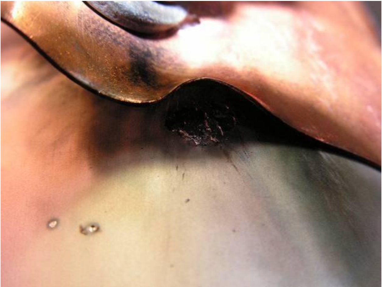
Fig. 8. 8/10µs 55kA surge current result on the flagstaff interconnection point between section and ground
