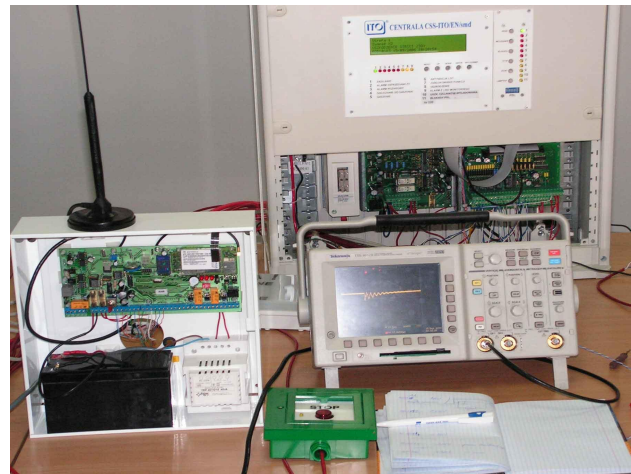
Fig. 1. Fire protection system during the EMC tests
